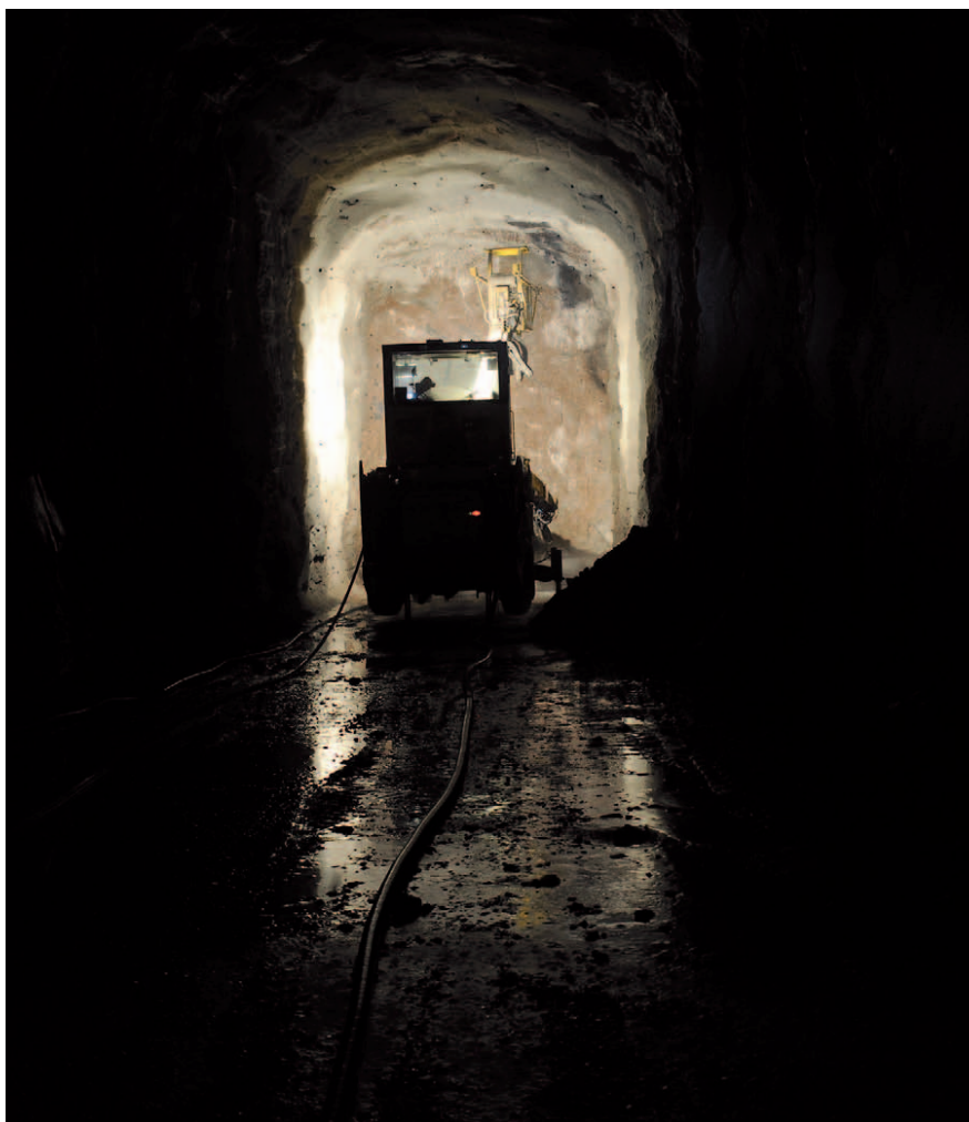
Excavation work at the connection tunnel of the VLJ Repository in Loviisa. Photo: Ari Haimi.
