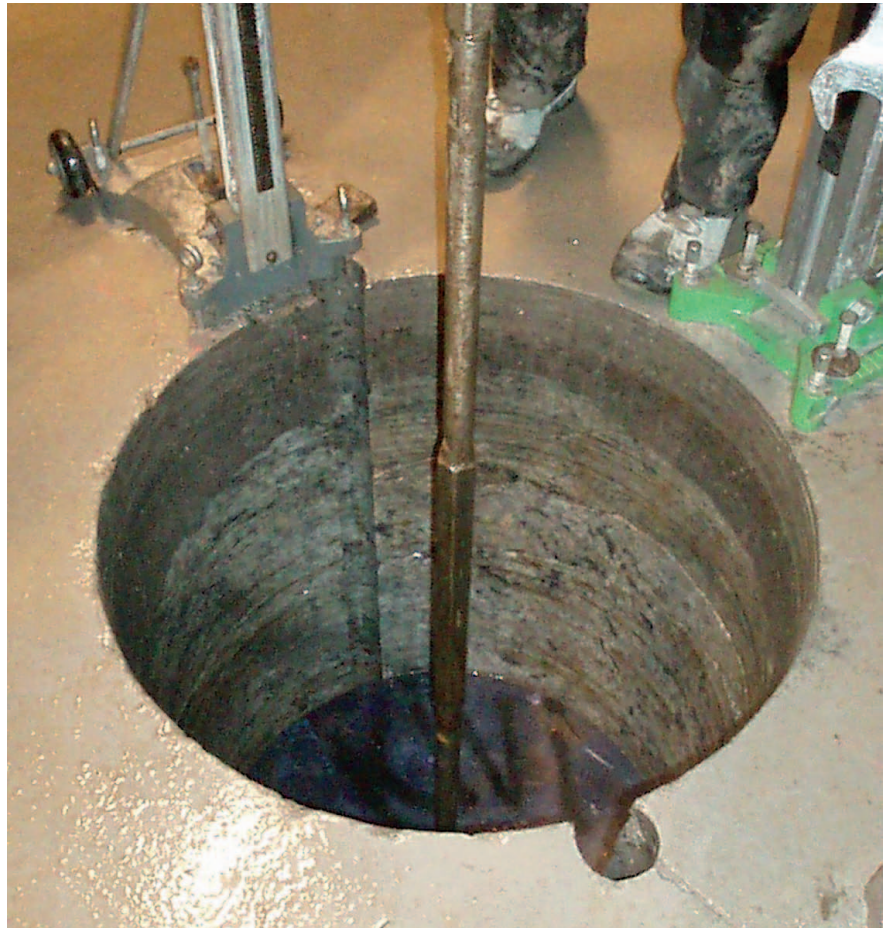
Drilling of a dia. 800 mm test hole in progress in Investigation niche 1.
